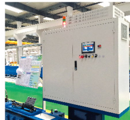
电控箱 Electric Cabinet
